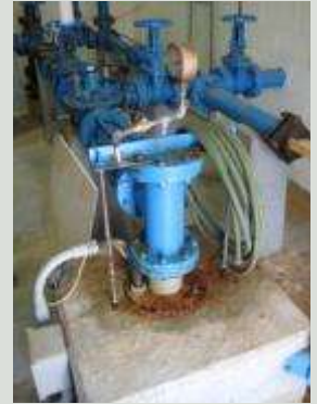
South Bruce, inside Pump house
