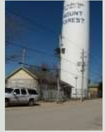
Well No. 3, booster pumping station and standpipe
